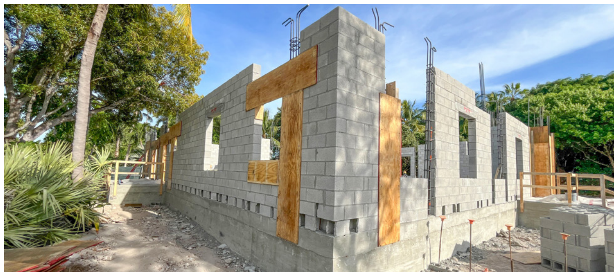
Work in progress at the future Grayvik Animal Center - Home of ORCAT.
